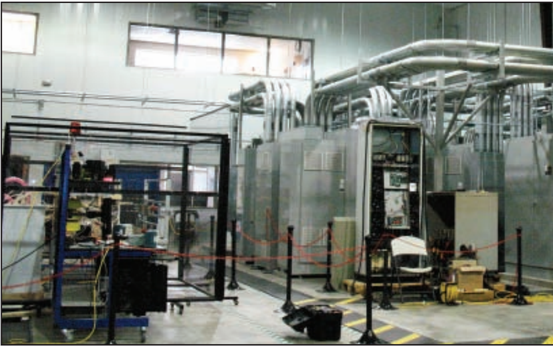
In 2009, NCREPT moved into a 7,000-square-foot world-class power electronics test facility in Fayetteville, Ark. The Center can work with experimental electricity distribution systems of up to 6.5 megawatts.
